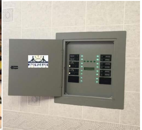
Smart Load Center—Outside
