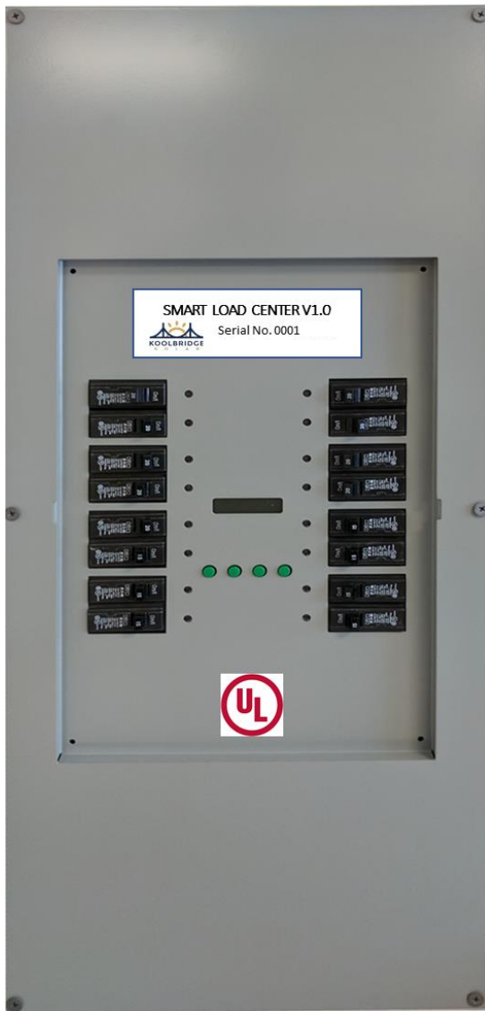
Koolbridge Solar SMART LOAD CENTER
